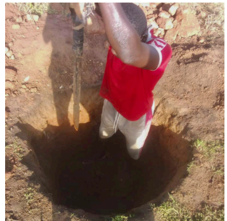
A Sunsang resident is pictured in December 2019 while constructing a household latrine. Photo: Alhassan Bukari
